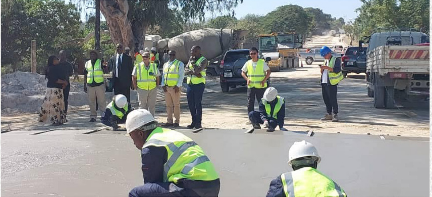
Minister of Infrastructure, Housing and Urban Development Hon. Eng. Charles L. Milupi, RDA Board of Directors Chairperson, Eng. Mulchand Kuntawala and the entourage inspect concrete works at Nayuma harbor.
