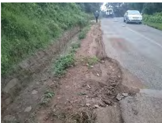
Figure 8-18: Poor – Gap between surfacing and drain lining
