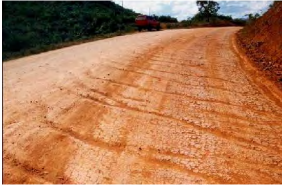
Transverse erosion in fine material
