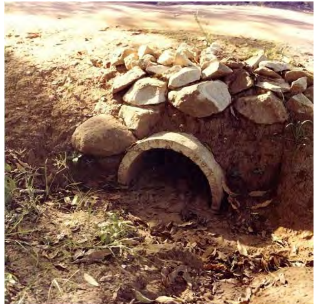
Figure 7-8: Siltation problems at culvert outlet
