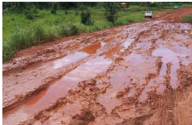
Figure 4-20: Typical road condition in a wet/marshy area
