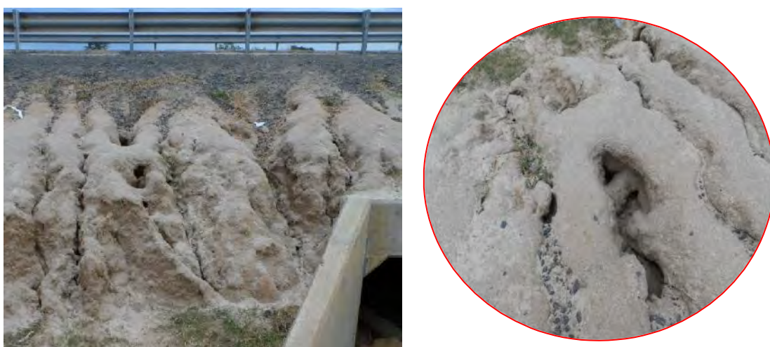
Figure 4-13: Piping in dispersive soils
