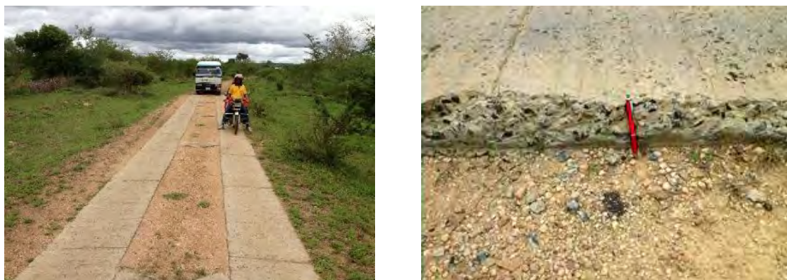
Figure 11-10: Concrete strip road with dangerous edge drop
