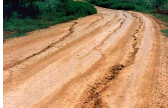
Longitudinal erosion in fine material
