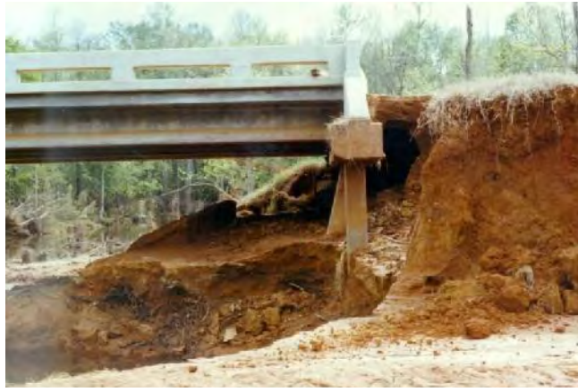
Figure 4-26: Typical bridge scour
