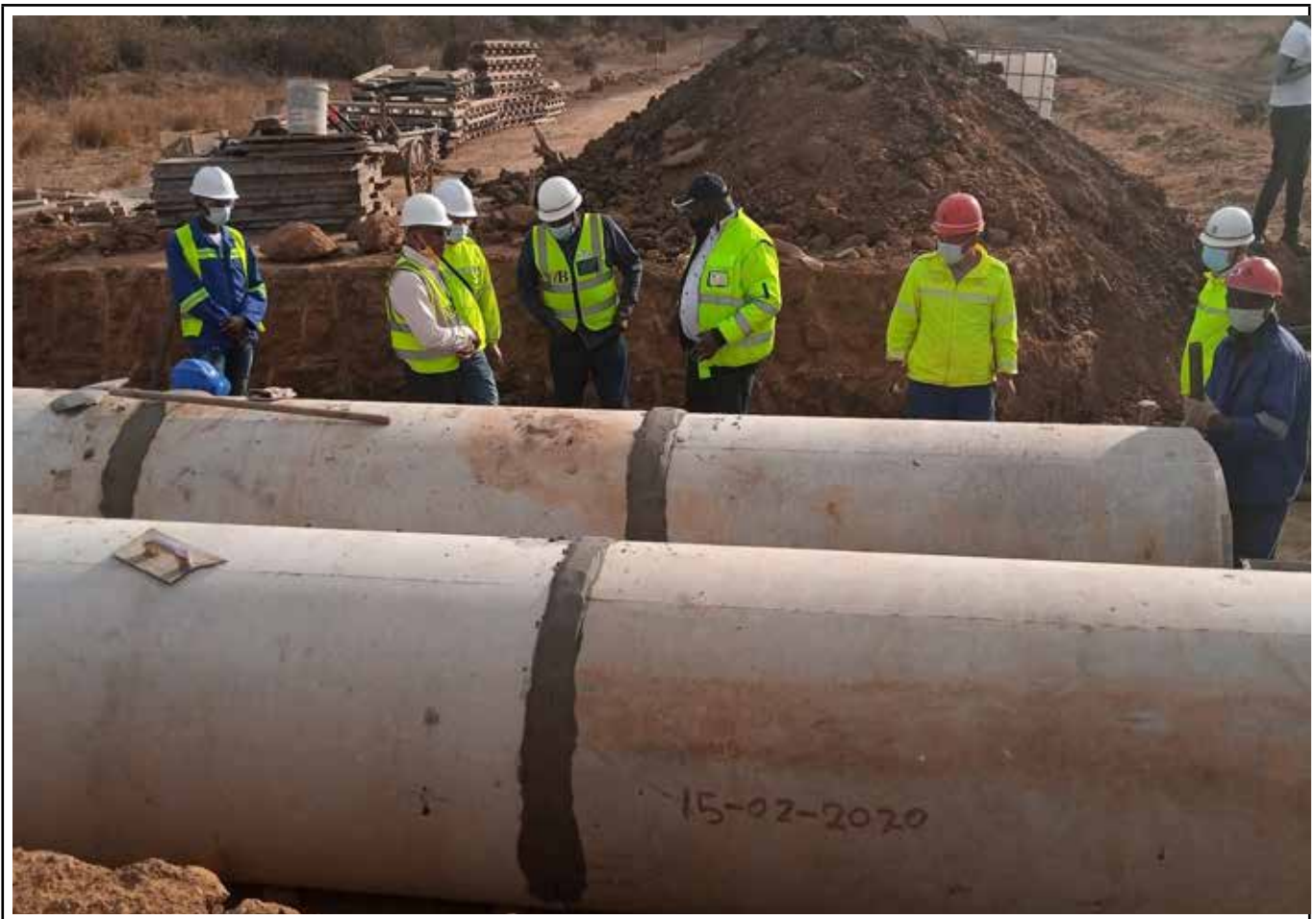
Figure 4: Installation of concrete culverts on Mumbwa Road under IRCP in Central Province.
