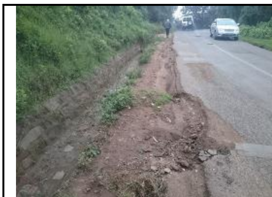
Figure 2-2: Bad – Gap between surfacing and drain lining
