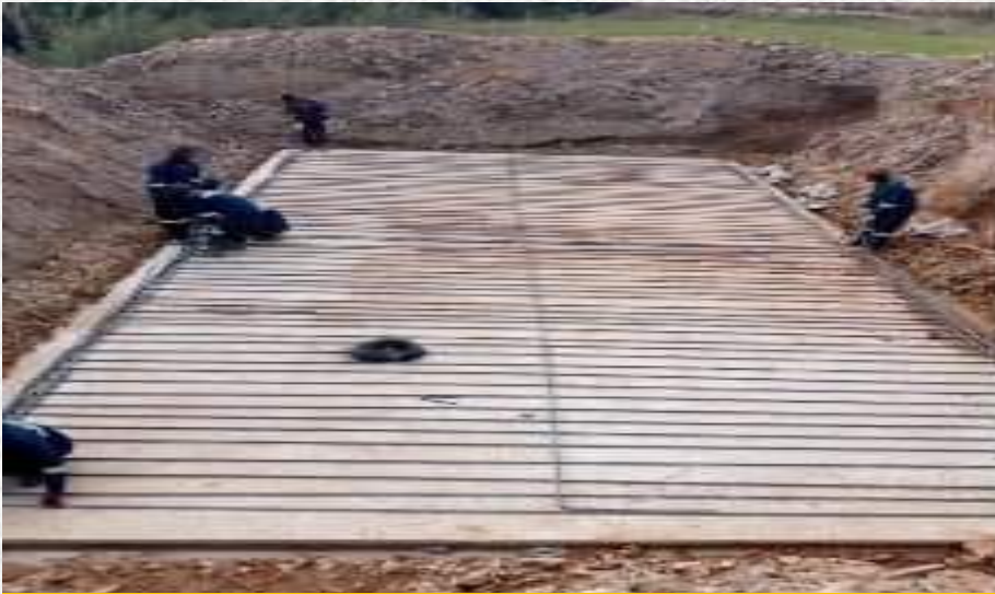
Tying steel reinforcement for the base at Lwitikila ACROW Bridge in Kanchibiya District.
