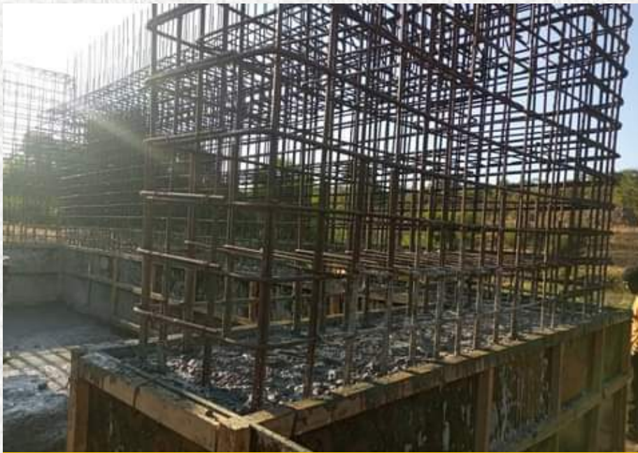
Formwork and casting of concrete for the abutment stem at Mkushi Bailey Bridge.
