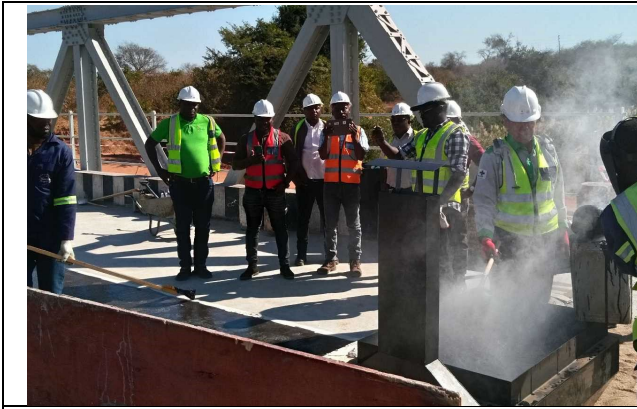
Photo of waterproof material dissolving
