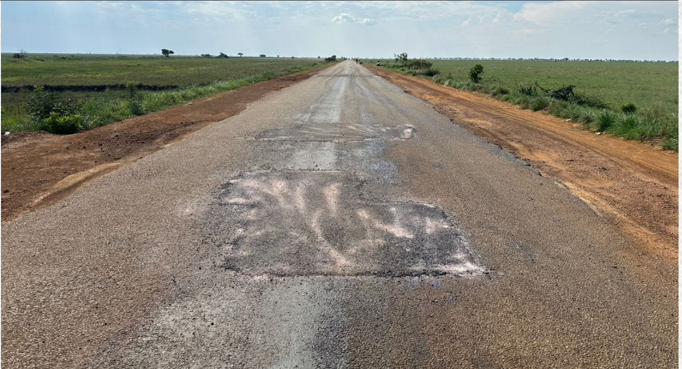
Patched sections on Tuta Road from Musaila-Mukuku Bridge.
