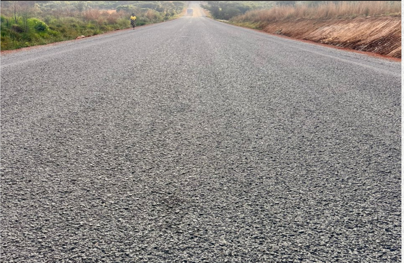
Reconstruction works on the damaged section of the Great North Road from Lukulu Bridge.
