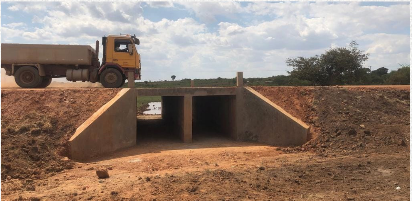
The Insitu Jeremiah box culverts along the Lundazi-Chasefu Road in Eastern Province.
