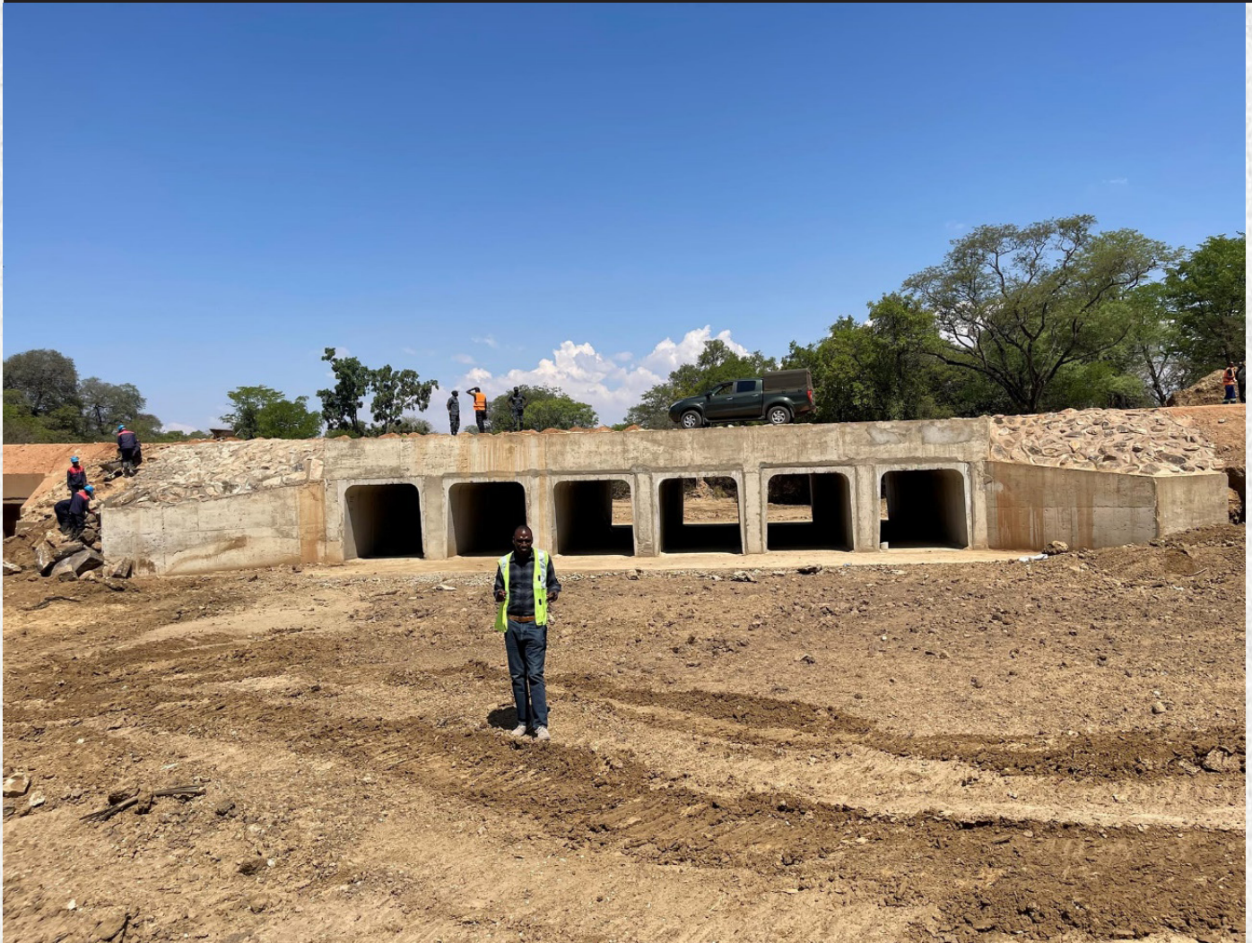
Six lines Dongo culvert along the Kalomo-Dundumwezi-Itezhi Tezhi Road in Southern Province.
