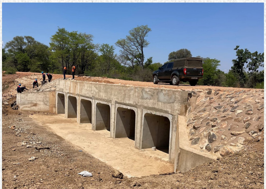
Six lines Dongo culvert along the Kalomo-Dundumwezi-Itezhi Tezhi Road in Southern Province.
