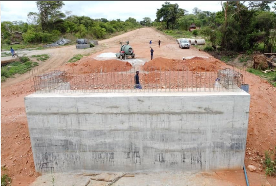
Construction of a Bailey Bridge in Luano District in Central Province underway.
