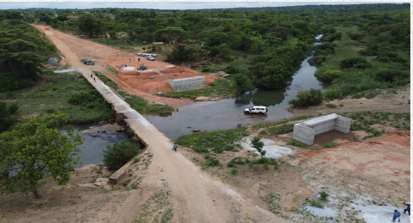
An aerial view of construction works at Mkushi Bailey Bridge in Luano District in Central Province.
