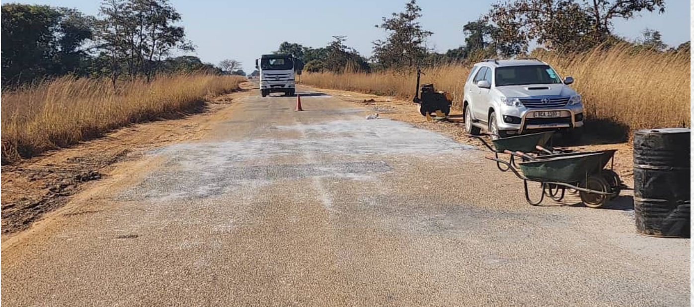
The patched section of the Tutu Road.
