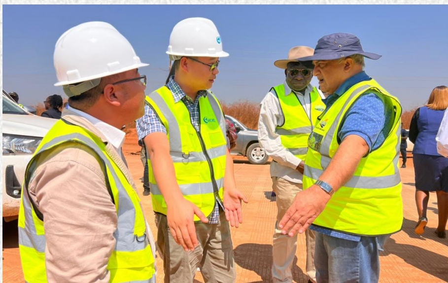
RDA Board of Directors Chairperson, Eng. Mulchand Kuntawala (far right) and Infrastructure, Housing and Urban Development Minister, Hon. Eng. Charles L. Milupi inspect the concrete section of the Chingola-Kasumbalesa Road rehabilitation project.
