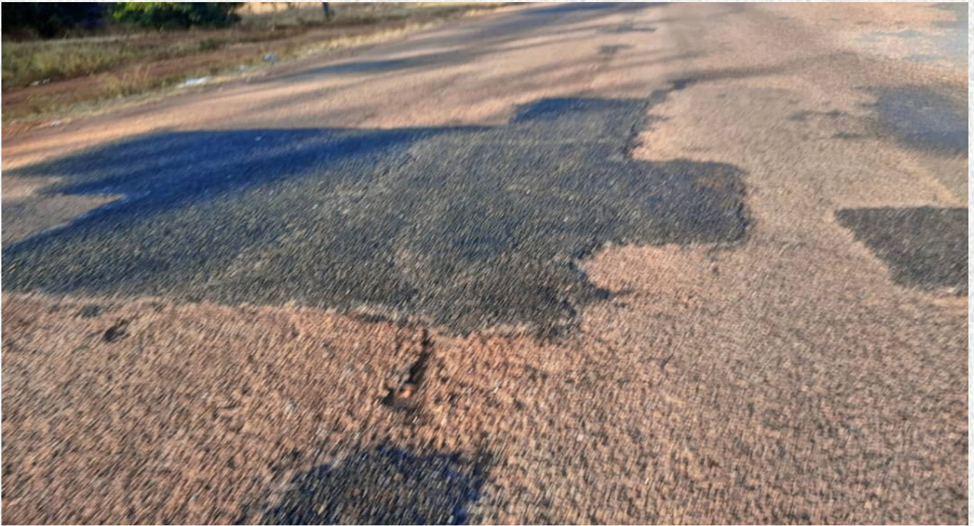
Patched section of the Chipata-Mfuwe Road.
