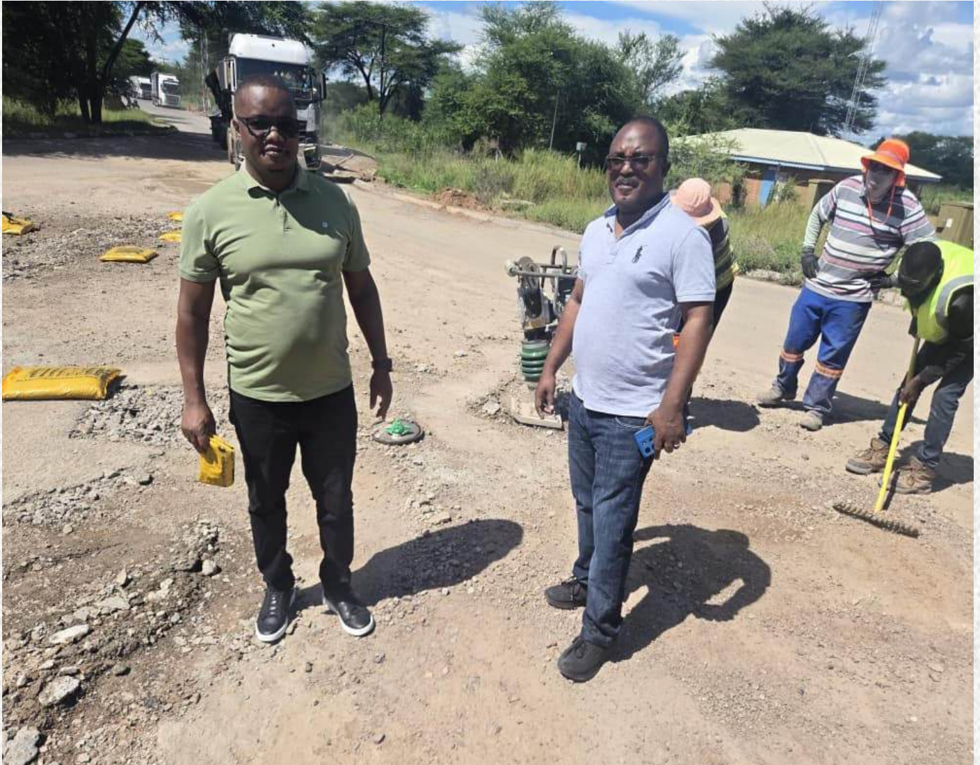
Acting Director-Road Maintenance, Eng. Paul Habasimbi and Acting Director-Construction and Rehabilitation, Eng. Chabala Pandeki during the inspection of pothole patching on the Kazungula-Kasane Road.
